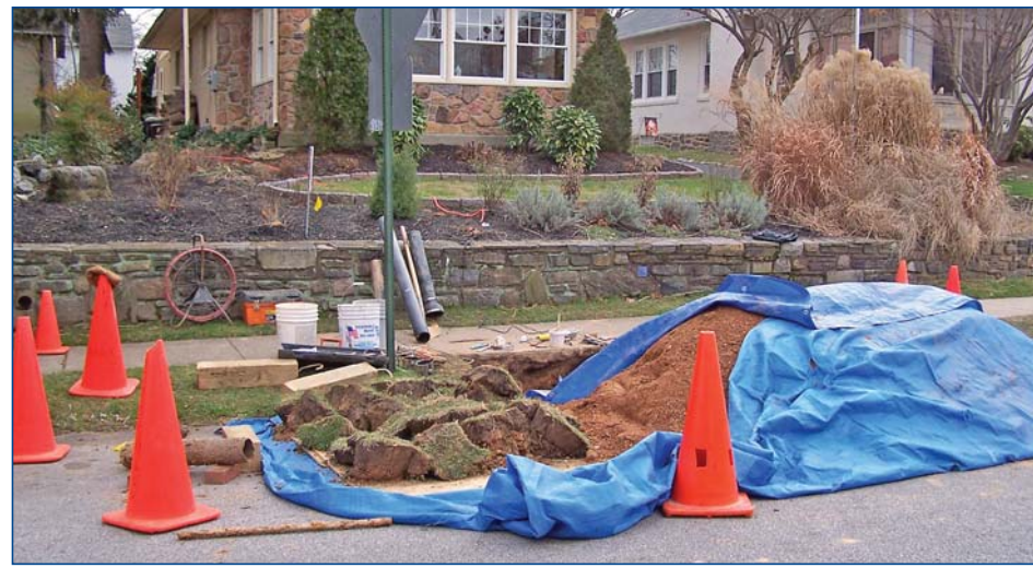
Carefully cut sod from a pit is stockpiled and kept moist during the job so that it can be replaced exactly as it was. This is one of many extra measures The Pipeshark takes to protect customers' lawns and trees.
