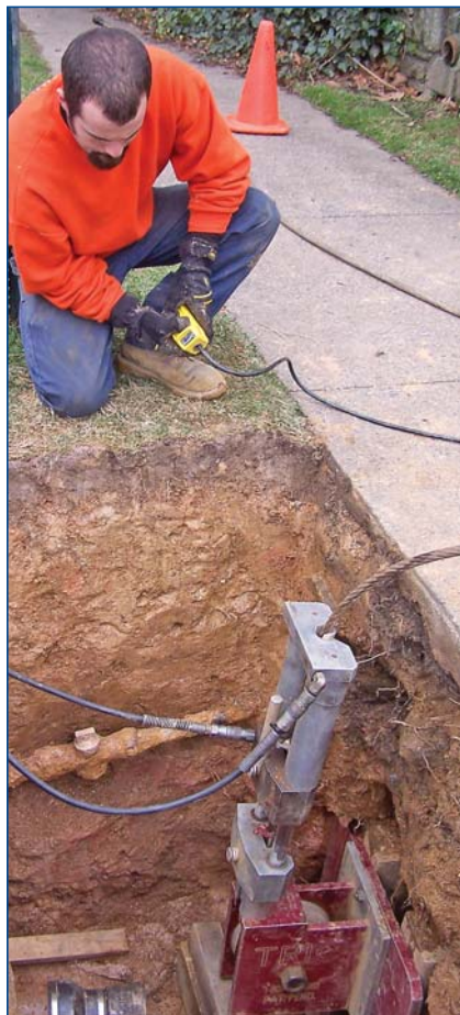
The Pipeshark technician Steve Helms operates the company's bursting unit, supplied by TRIC Tools.
